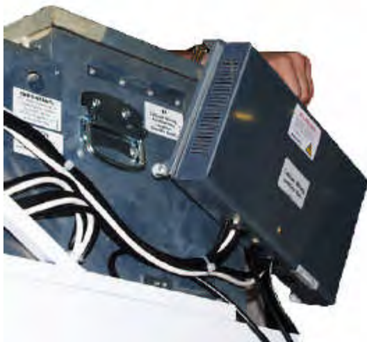
Figure 7: Cabinet Wiring Junction Box
